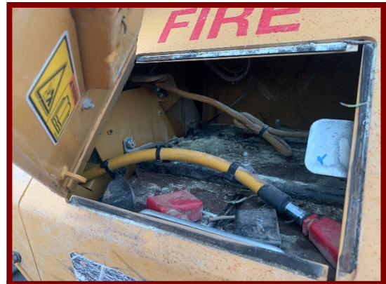
Picture 3: Battery box where the fire was first observed by the operator.
