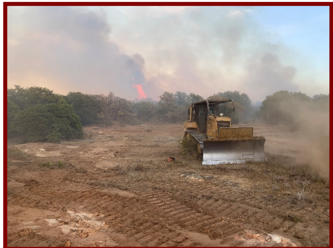
Picture 1: The disabled dozer after the engine compartment fire was suppressed.
